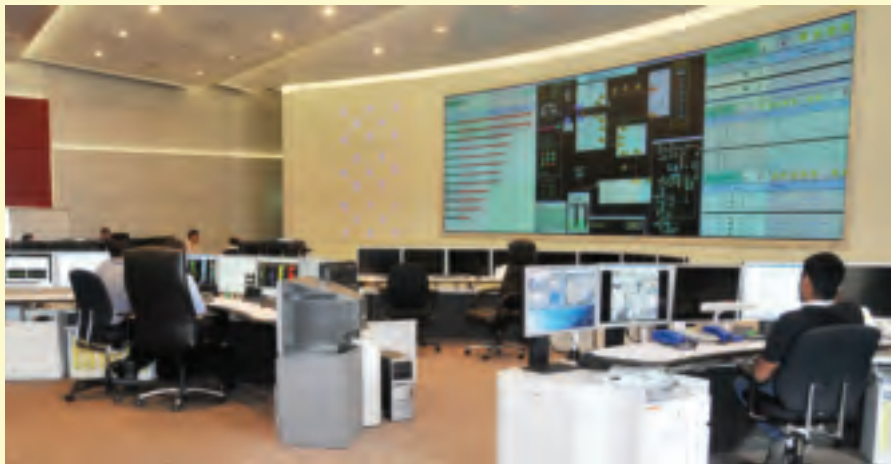
TNB's National Load Despatch Center
