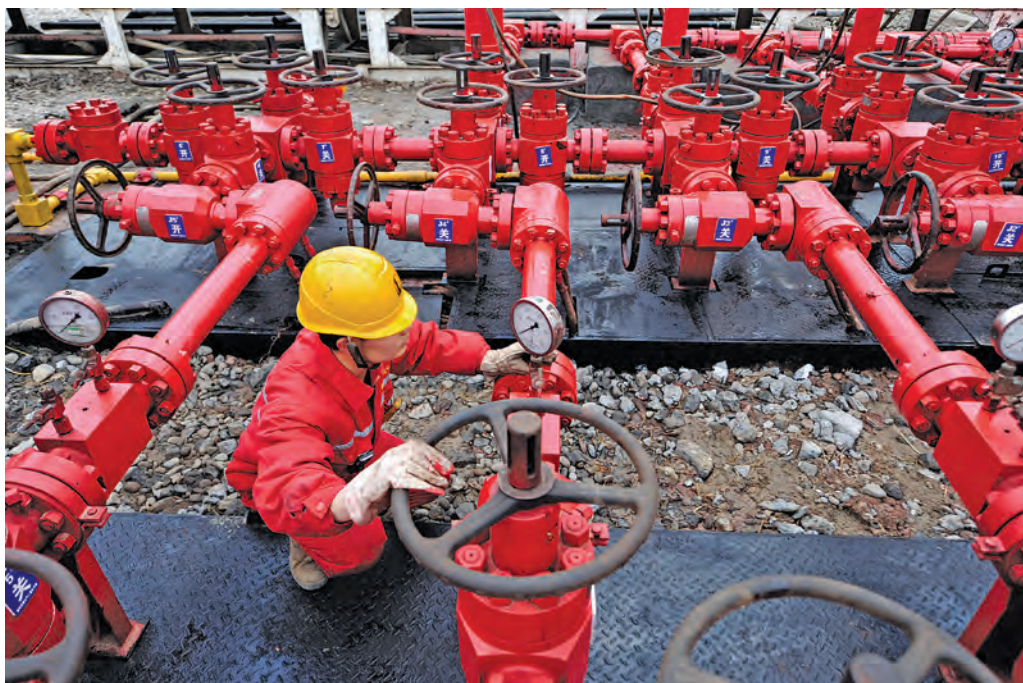
Pipe dreams: a natural gas well in Sichuan, China, November 2013
